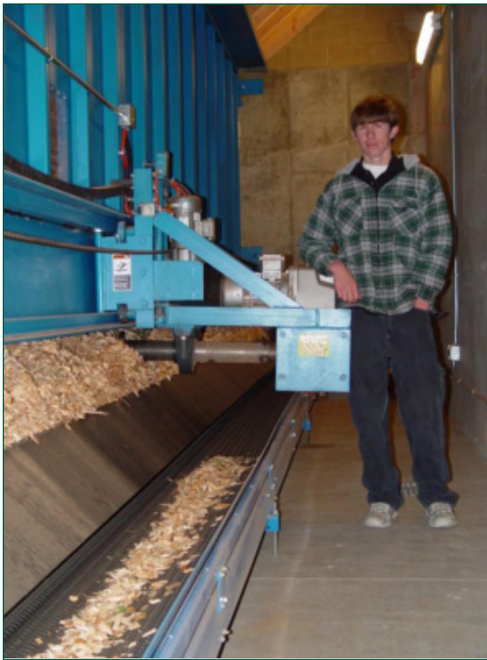
Wood chips ride a conveyor to Darby School's new biomass boiler. This alternative reduces school heating costs and effects associated with open burning of excess forest fuels. (Photo courtesy of USDA Forest Service.)
