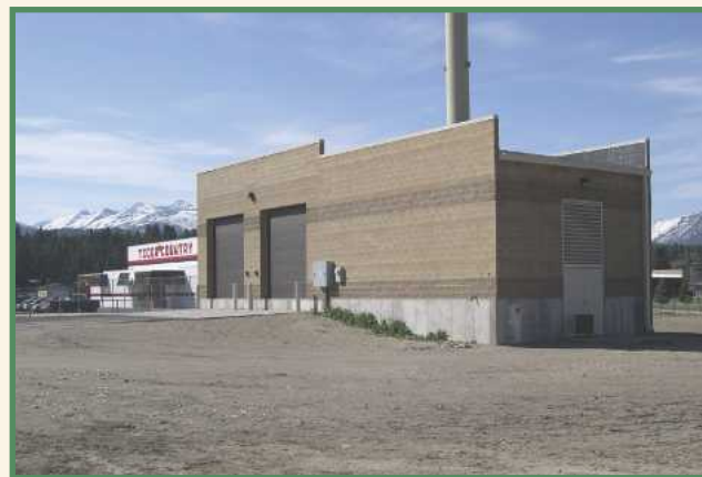
Figure 2. — This biomass-fueled boiler facility provides heat for multiple school buildings in Montana.
