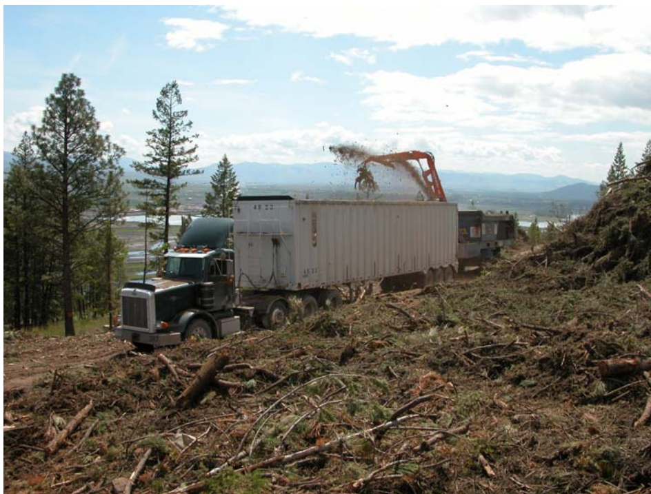
Figure 4. Loading chip van parked on forest road. 120 CY chip van shown.
